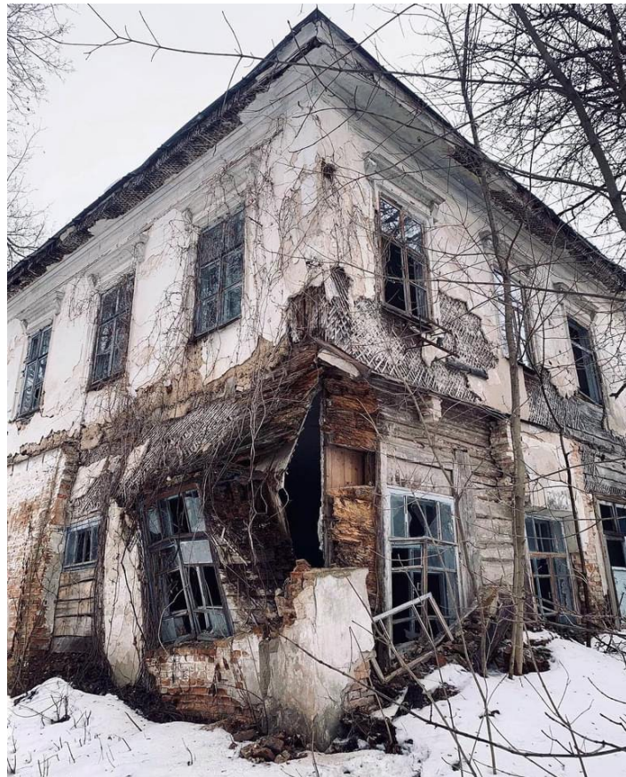
Figure 42 - Homutetz damage on main house
